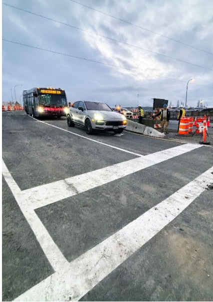
Figure 1: The first vehicles to travel over the new Phase 1 overpass following the westbound traffic switch on January 16, 2025.
